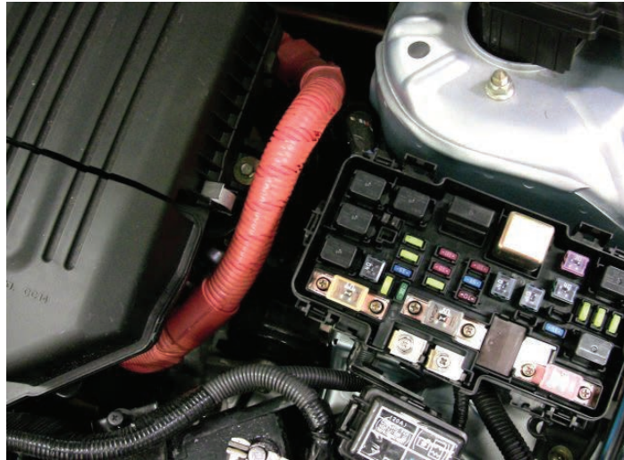
Figure 17.63 Power cable connected to the motor (remember, orange cables are high voltage)
